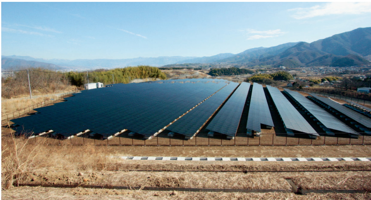
10 MW Komekurayama Solar Power Plant, (Kofu City, Yamanashi Prefecture), Owner: TEPCO (Tokyo Electric Power Company)
