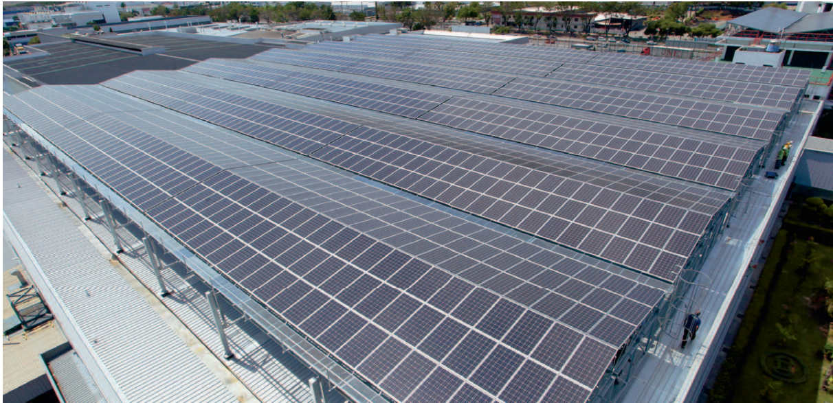
BIPV System at Bosch plant, Penang, Malaysia
