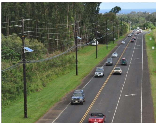
Kauai Island Utility Cooperative Utility Pole Mounted PV Panels (Courtesy: Kauai Island Utility Cooperative)
