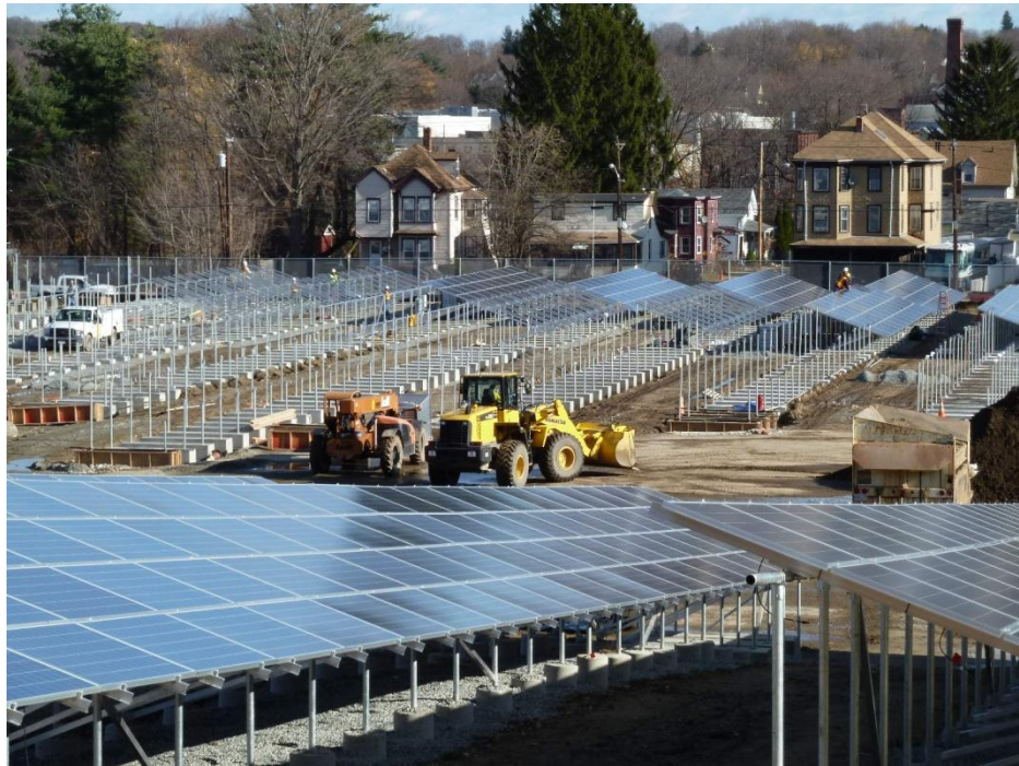
National Grid's Utility-owned Haverhill Solar Project (Courtesy: National Grid)
