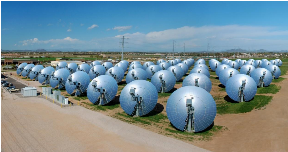
Salt River Project 1.5 MW Maricopa CSP Project (Courtesy: Sterling Energy Systems)
