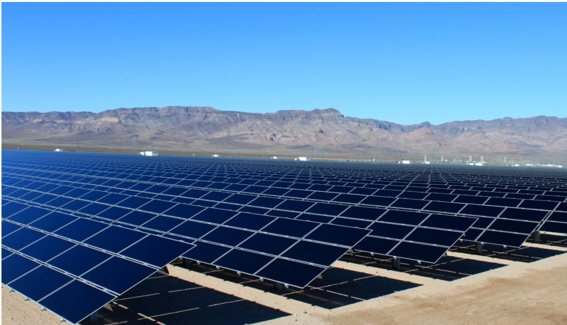
Pacific Gas and Electric 48 MW Copper Mountain PV project (Courtesy: Sempra Generation)
