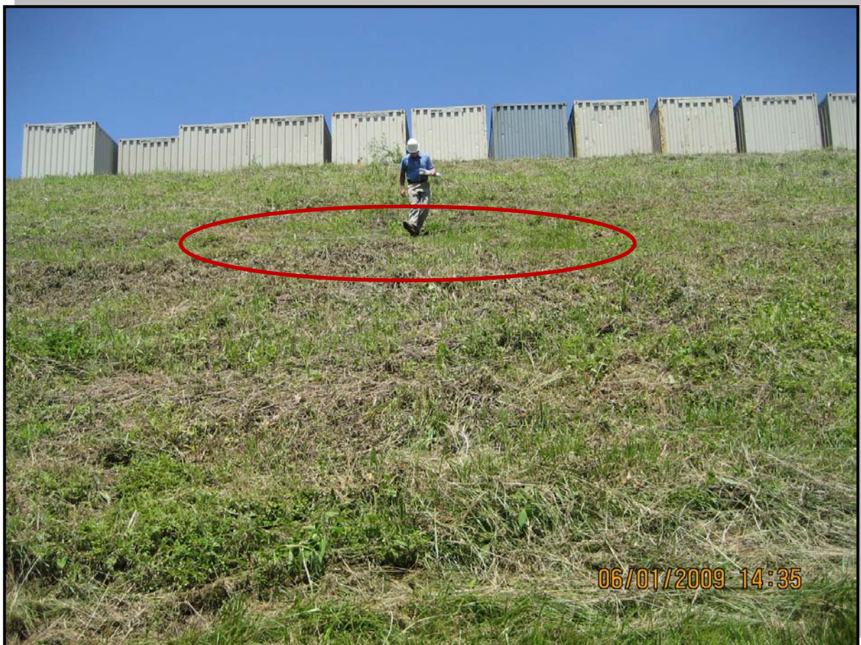
Photo 10 – Old slough on western downstream slope
