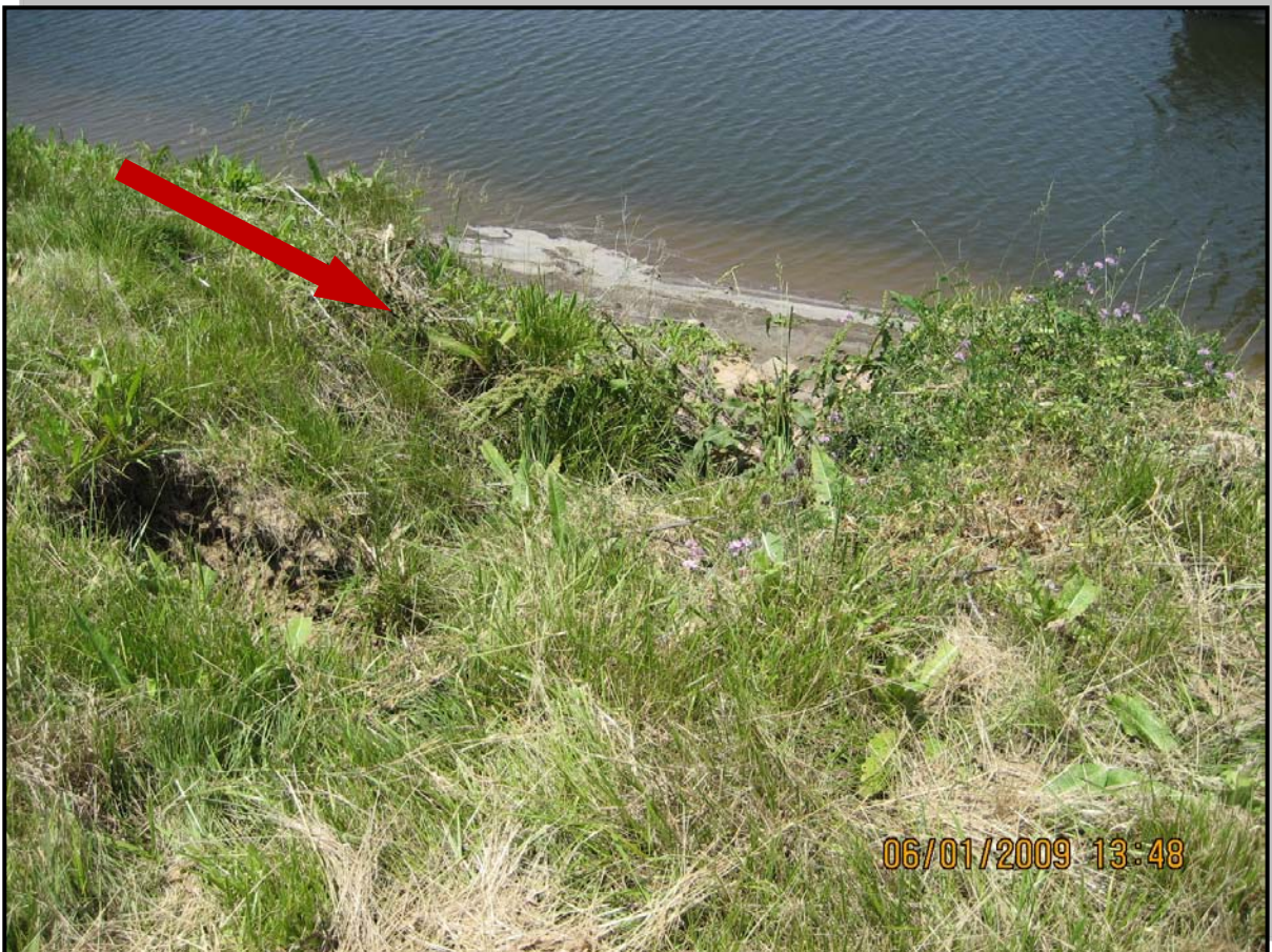
Photo 4 – View of typical erosion gullies in freeboard area along upstream slope near Floating Dock
