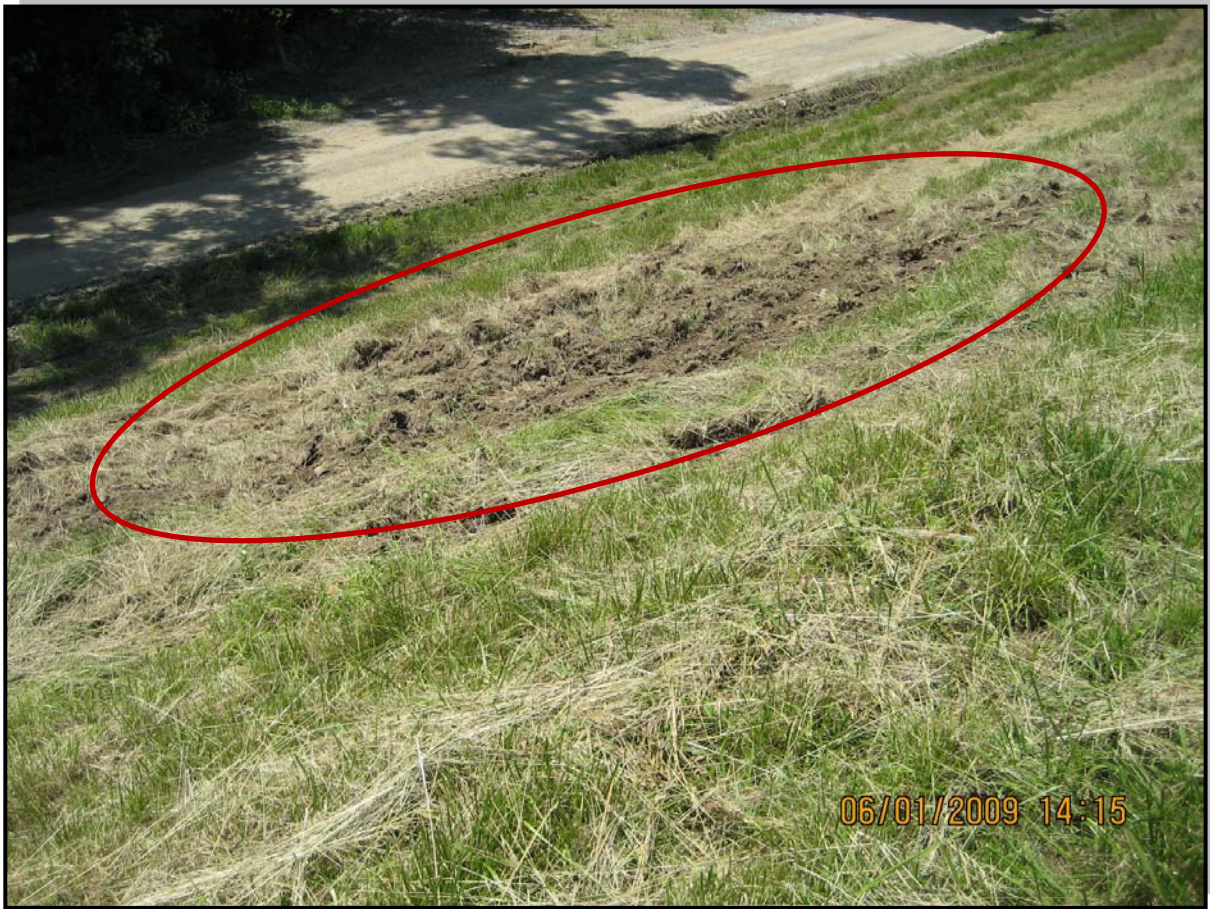
Photo 9 – Typical rutting and slope sloughing due to heavy mowing tractor, western downstream slope
