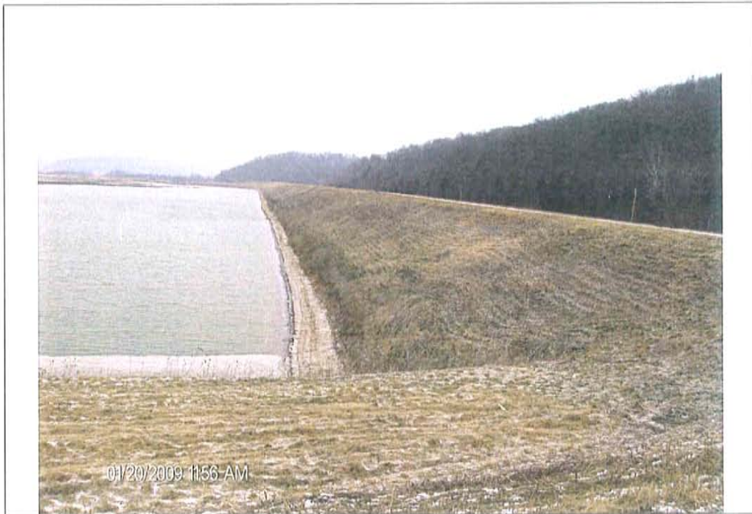
Photo #1: Wave erosion, East embankment, downstream slope, looking North
