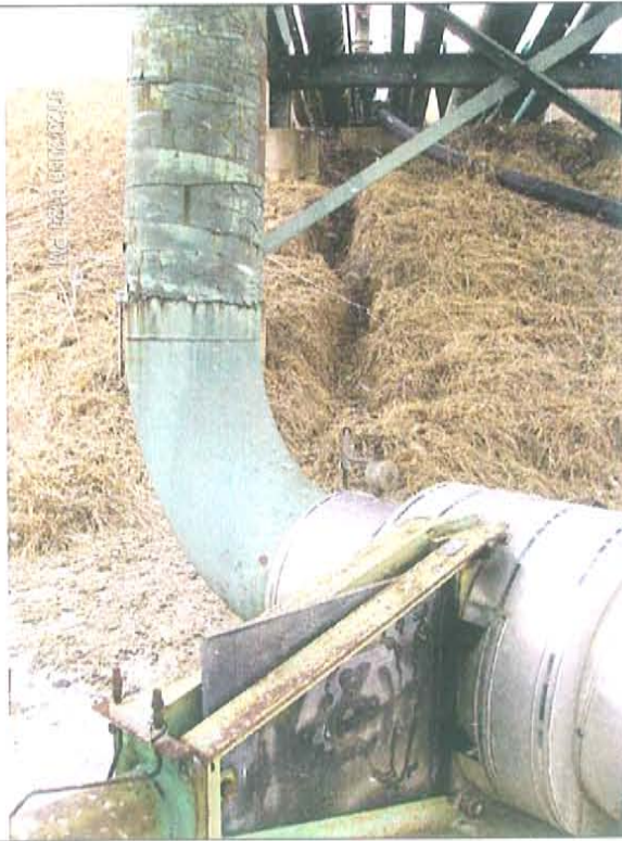
Photo #10: Minor erosion below piping, South embankment downstream slope
