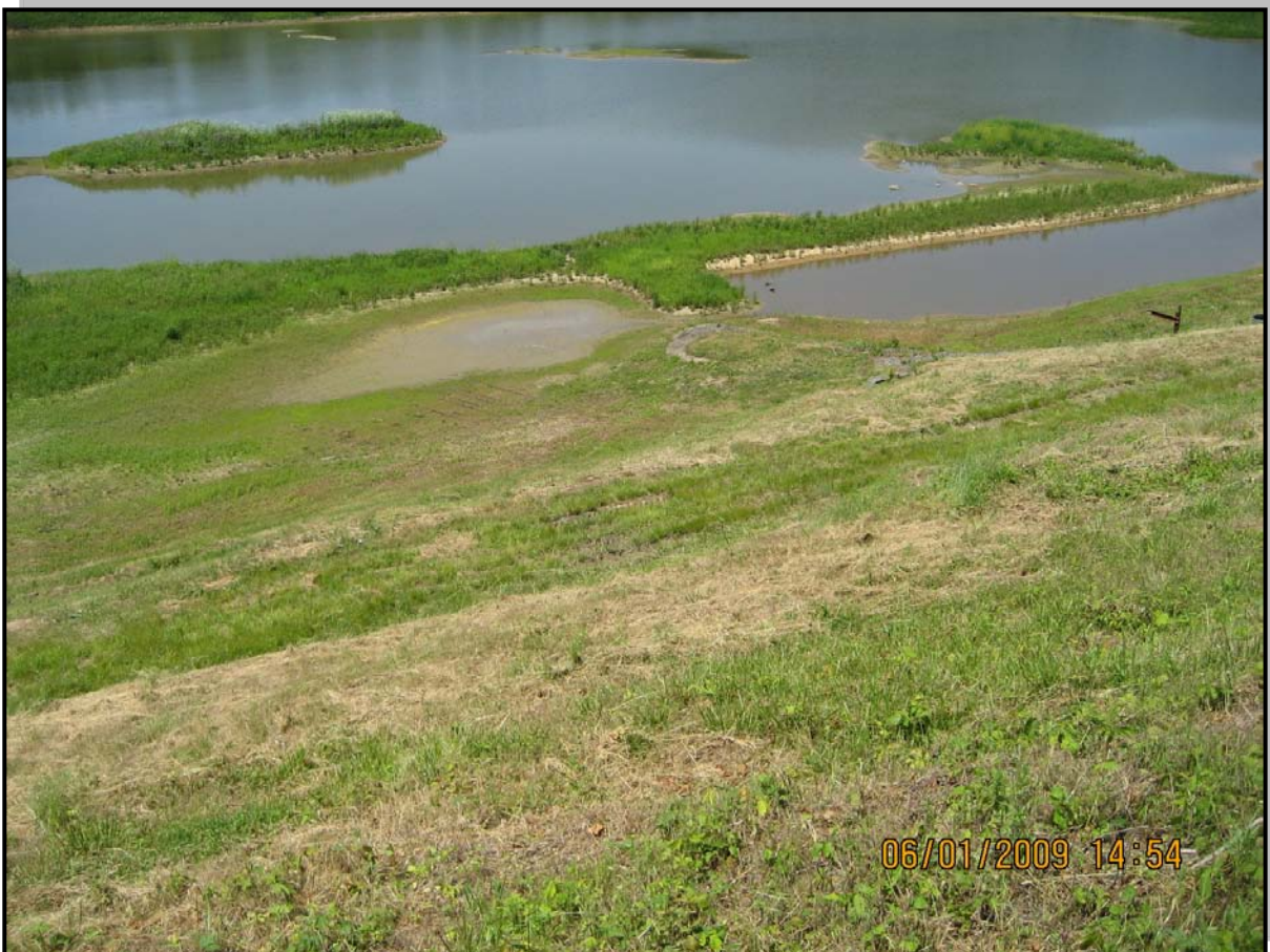
Photo 12 – View of Emergency Fly Ash Pond and northern slope of Bottom Ash Pond
