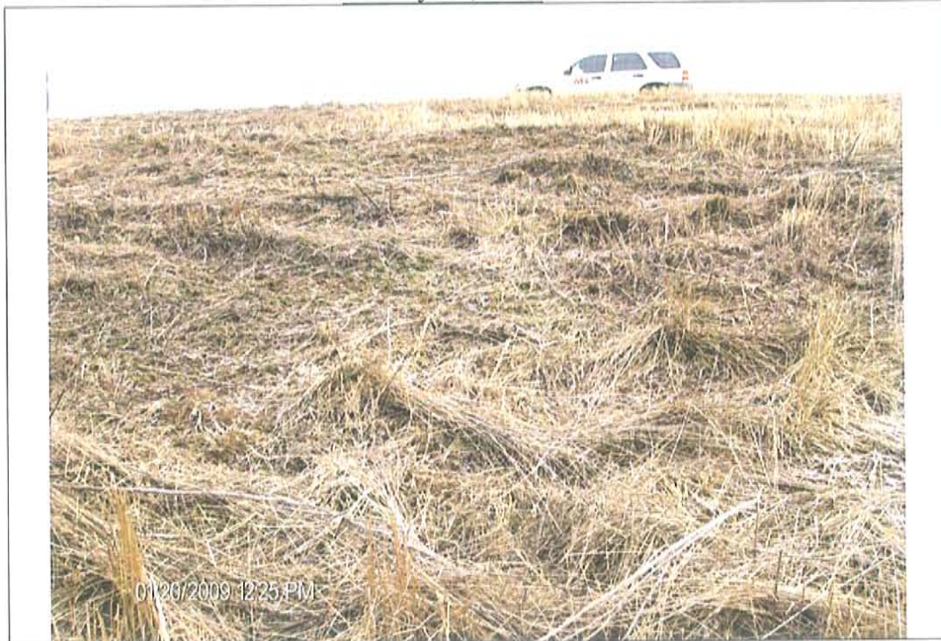
Photo #7: Old slough, East embankment, downstream slope, looking East near NE corner of pond
