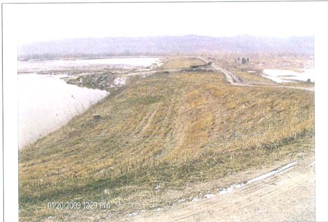
Photo #8: North embankment(shared dike with emergency ash pond), upstream slope, looking West
