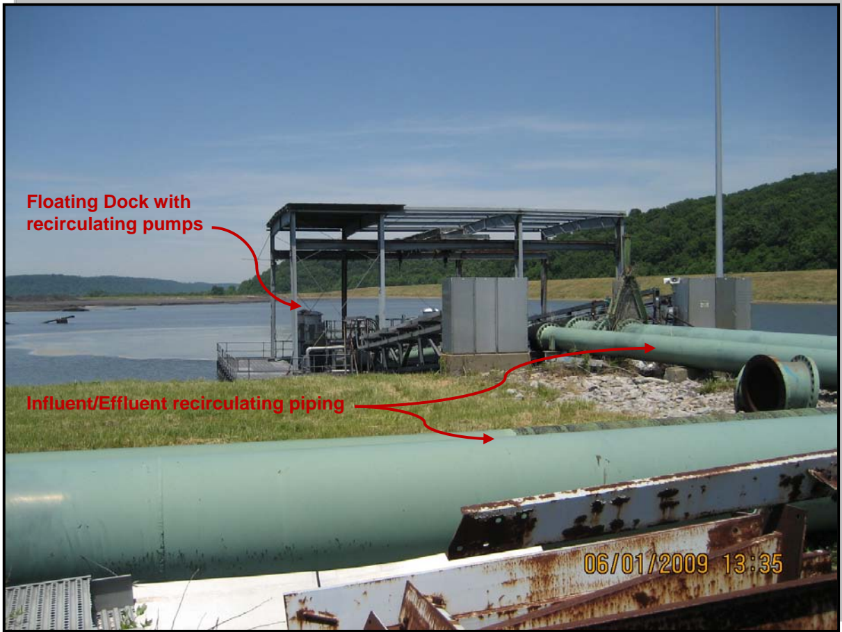
Photo 1 - View of Floating Dock with recirculating pumps and piping along South Dike
