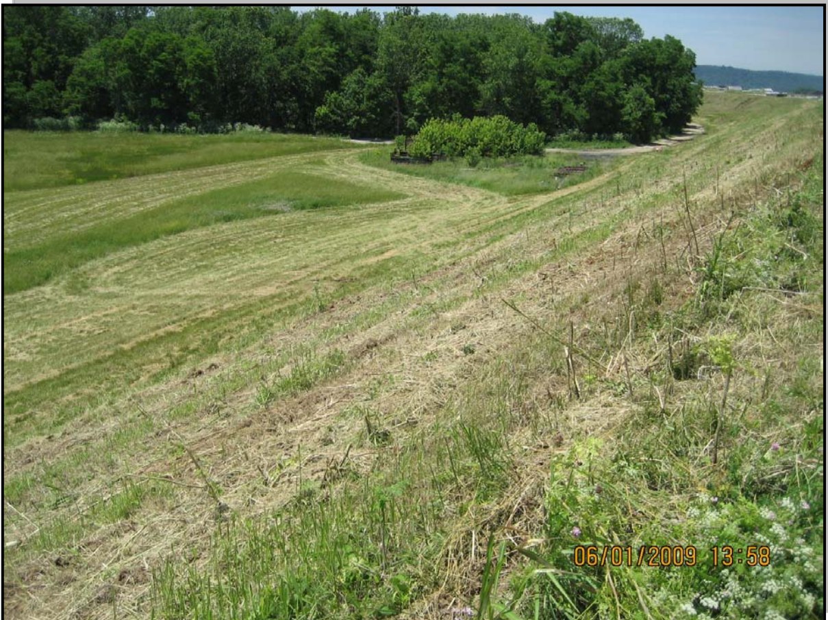
Photo 6 – Overview of downstream slope of the west dike from crest of south dike
