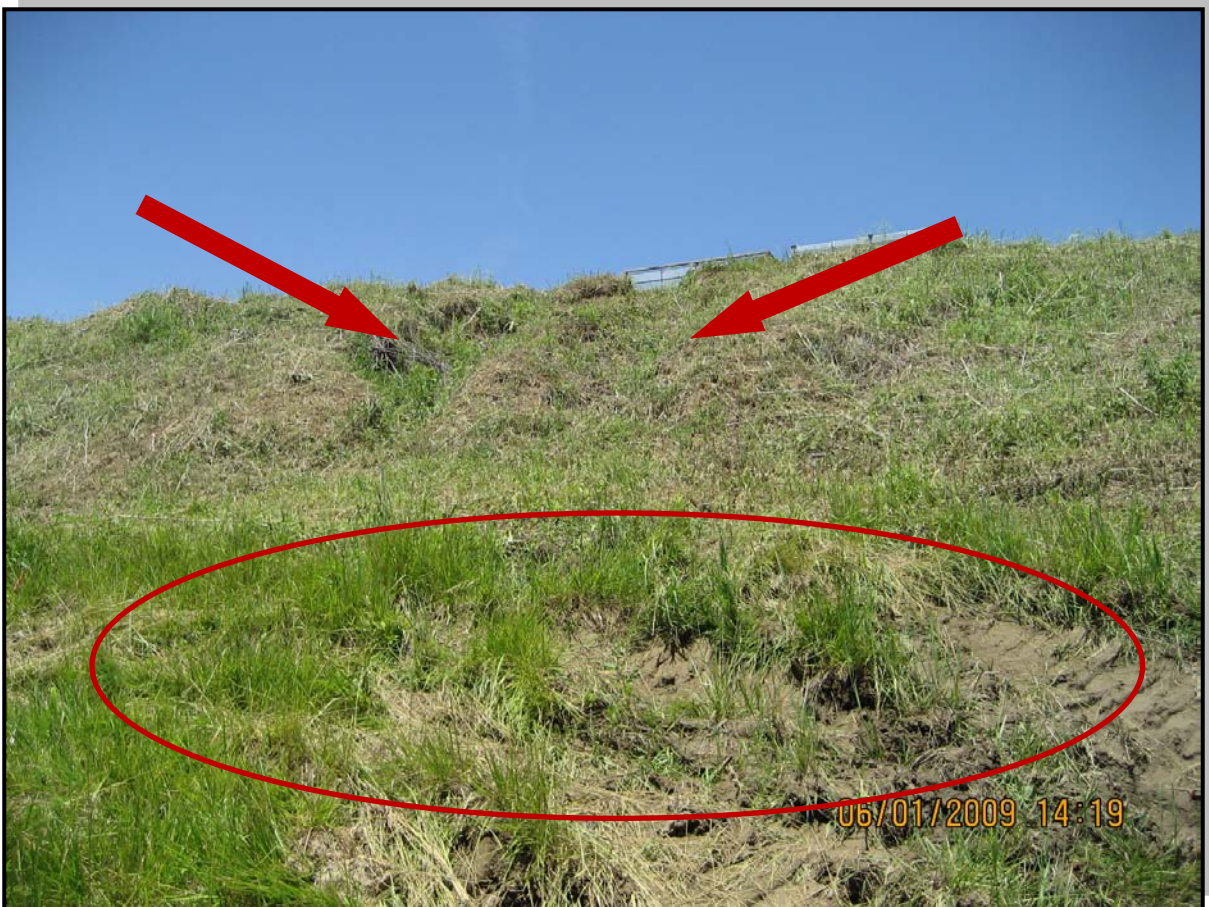
Photo 8 – Typical erosion gullies along western downstream slope near inside curved slope of embankment
