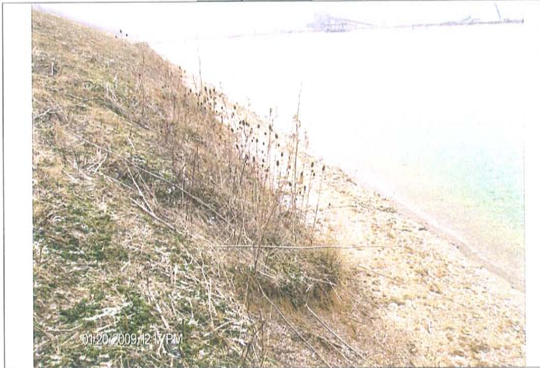
Photo #5: Wave erosion, steep drop near water surface, East embankment, upstream slope, directly across from bottom ash reclaim, looking South
