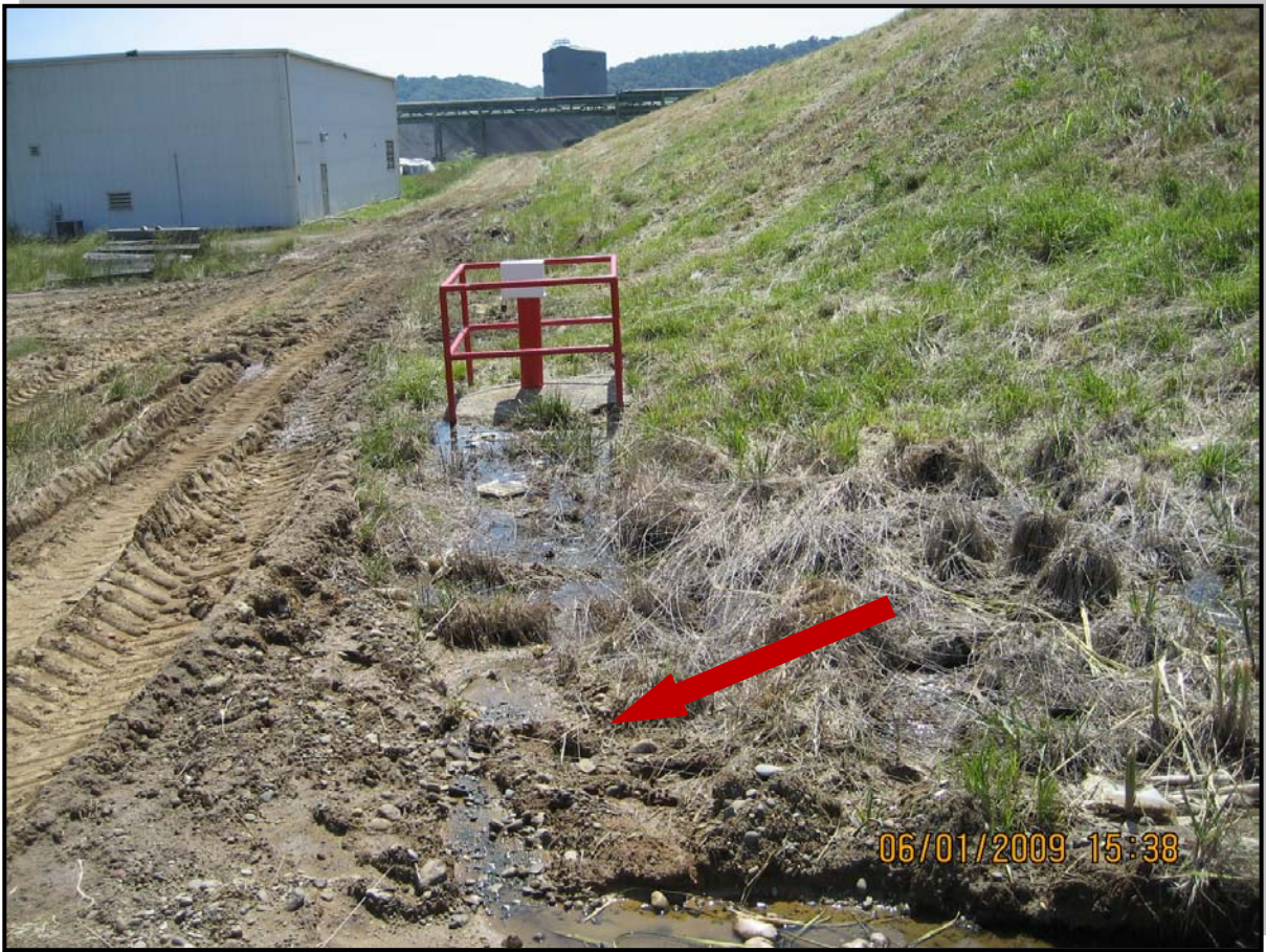
Photo 15 – Wet Area or minor seepage at toe of south embankment possibly due to discharge from gravel toe drain (View looking west)
