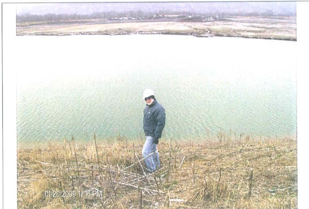
Photo #6: Appears to be filled in gully, East embankment, upstream slope, directly across from bottom ash reclaim, looking West
