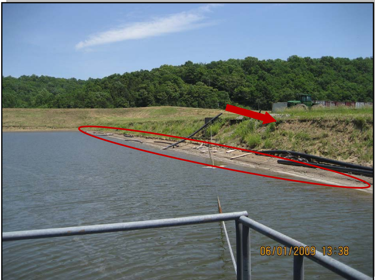
Photo 2 – View of South Dike with erosion and sloughing of upstream slope freeboard caused by wave action
