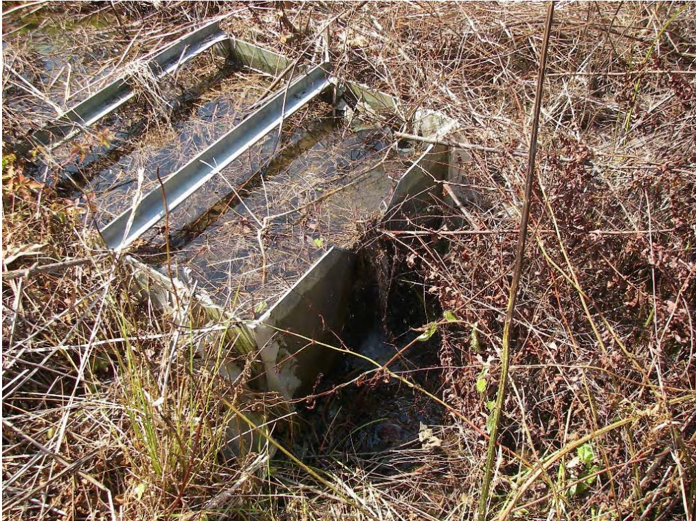
PHOTO 18: OVERGROWN SEEPAGE MEASUREMENT WEIR
