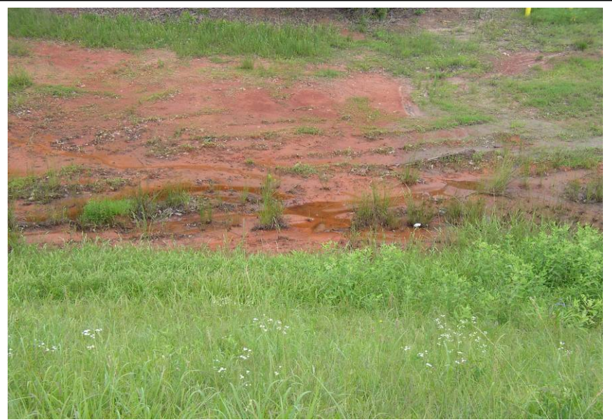
#67 Erosion at Downstream Slope of North Dike
