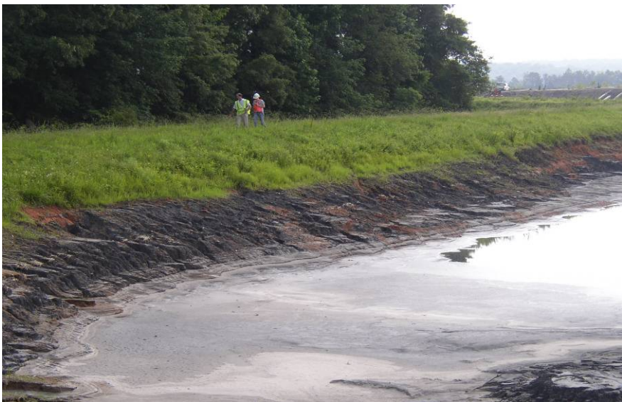
#73 Cell 1 Partially Excavated Ash on Upstream Side of Dike – Note Surface Erosion on Dike Slope
