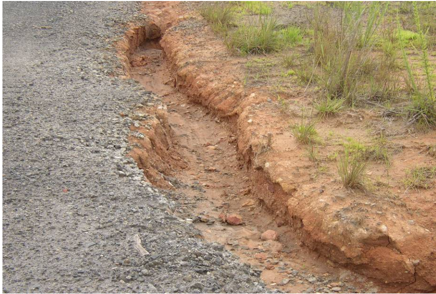
#76 Erosion Adjacent to Road Along Downstream Toe of North Dike
