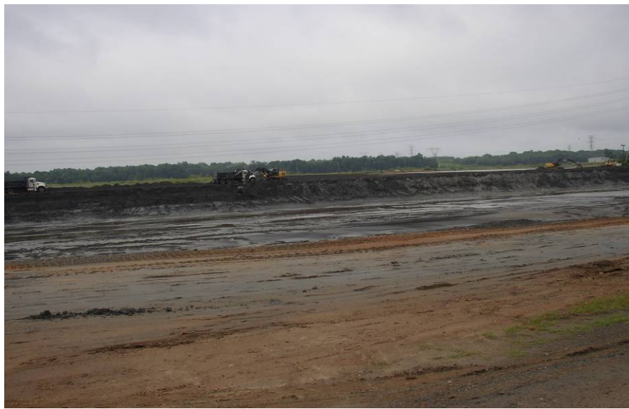
#57 Cell 3 Excavated to About 20-Foot Depth. No Water Impounded Due to Dewatering by Pumping.
