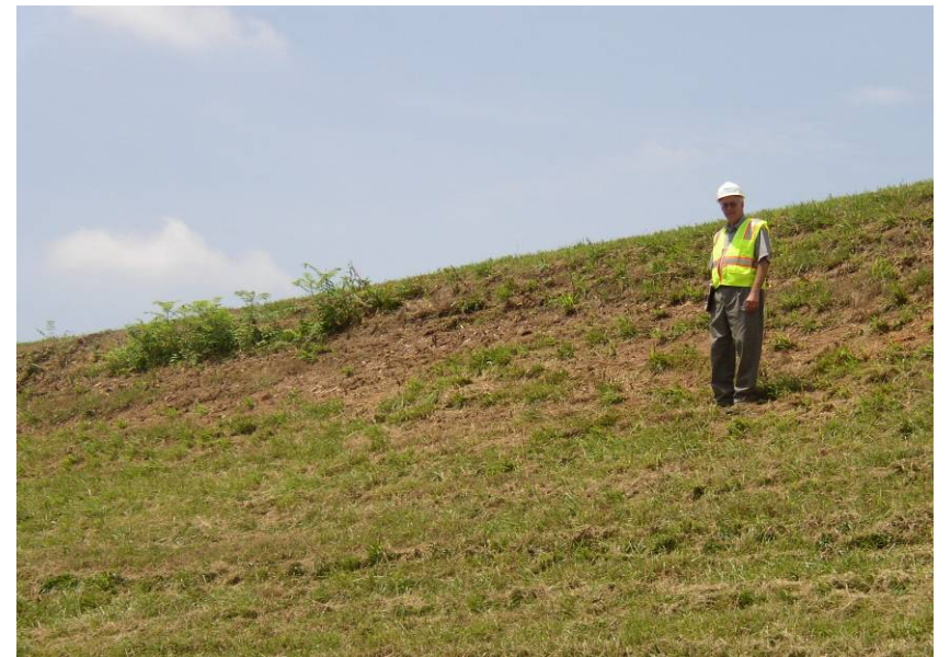
#25 Scarp on Upper Portion of Downstream Slope of East Dike
