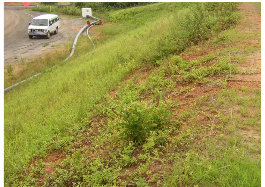
#66 Local Erosion Near Crest of North Dike
