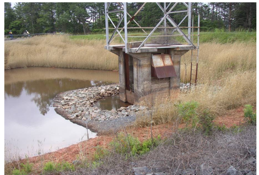
#55 Drop Inlet for Retained Ash Basin
