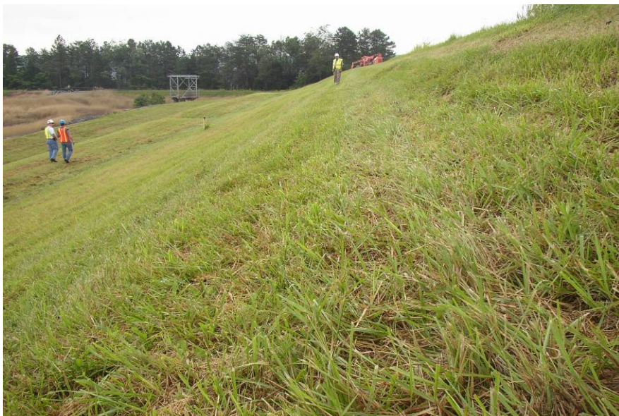
#54 Downstream Slope of North Dike (Note Evidence of Prior Scarps)
