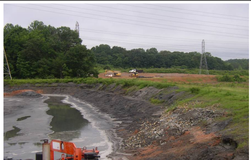
#63 Western Bend in North Dike at Cell 1 - Note Erosion in Upstream Slope of Ashfill
