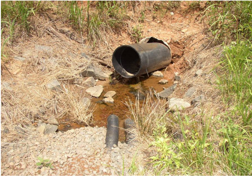
#35 Seepage Collection Area Near Maximum Section of Downstream Toe of East Dike
