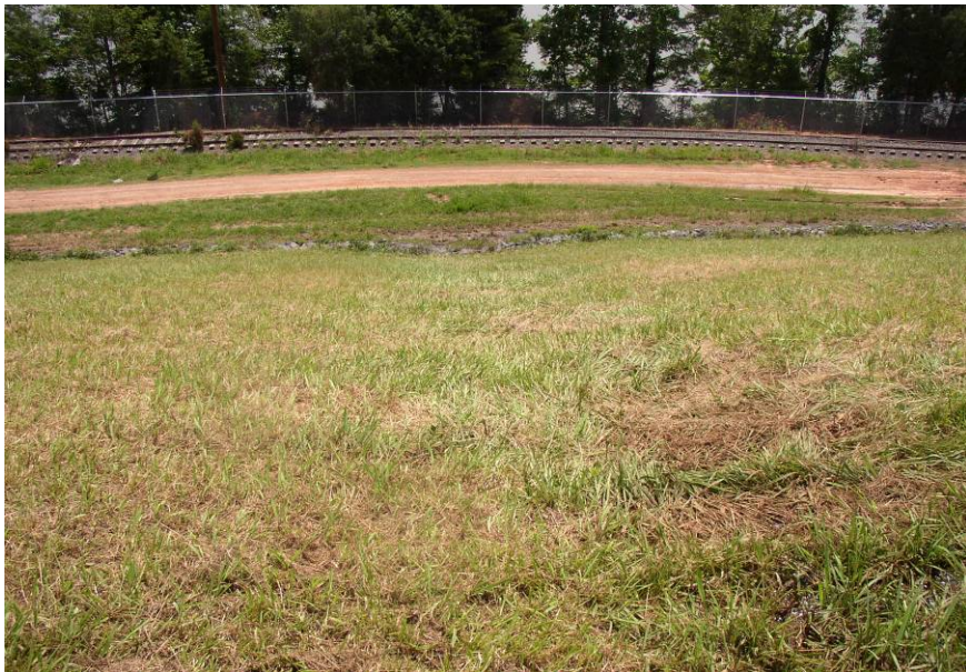
#24 Note Seepage/Ponded Surface Water at Downstream Toe of North Dike
