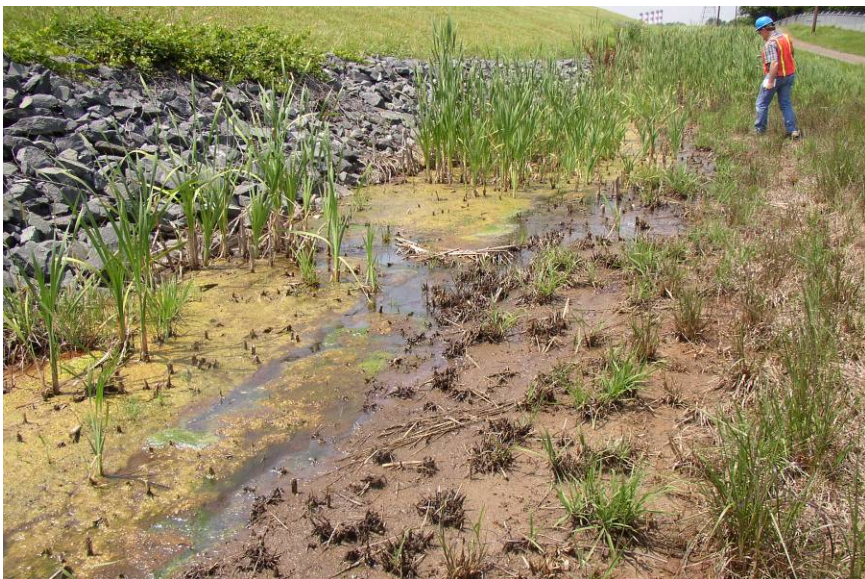
#36 Local Minor Seepage & Standing Drainage Flow at Downstream Toe of South End at East Dike
