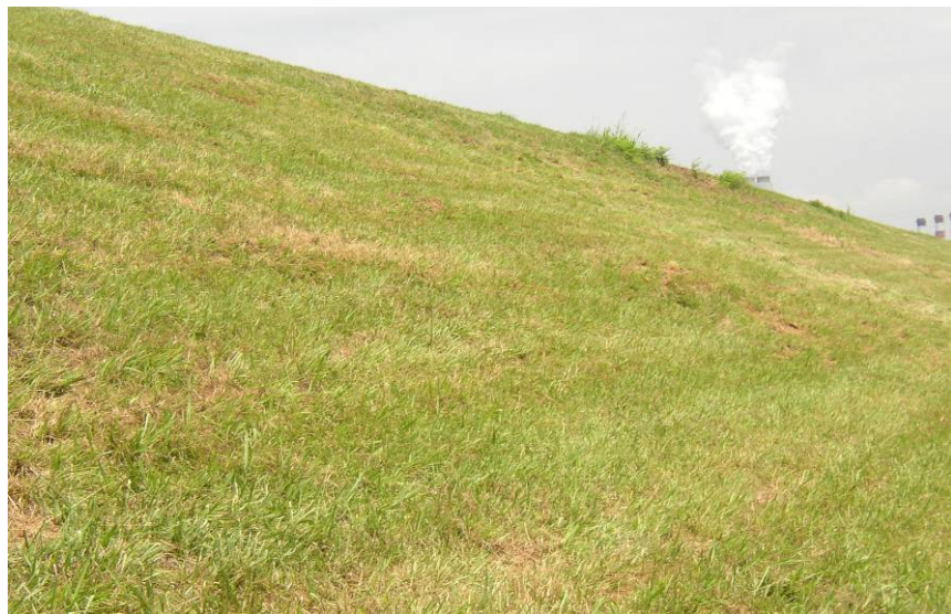
#27 Note Minor Bulging of Lower Portions – Upper Slope Above Stability Berm of East Dike
