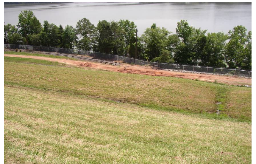
#13 Eroded Area of Downstream Toe Road from Operations due to Installation of Chain Link Fencing and Mowing
