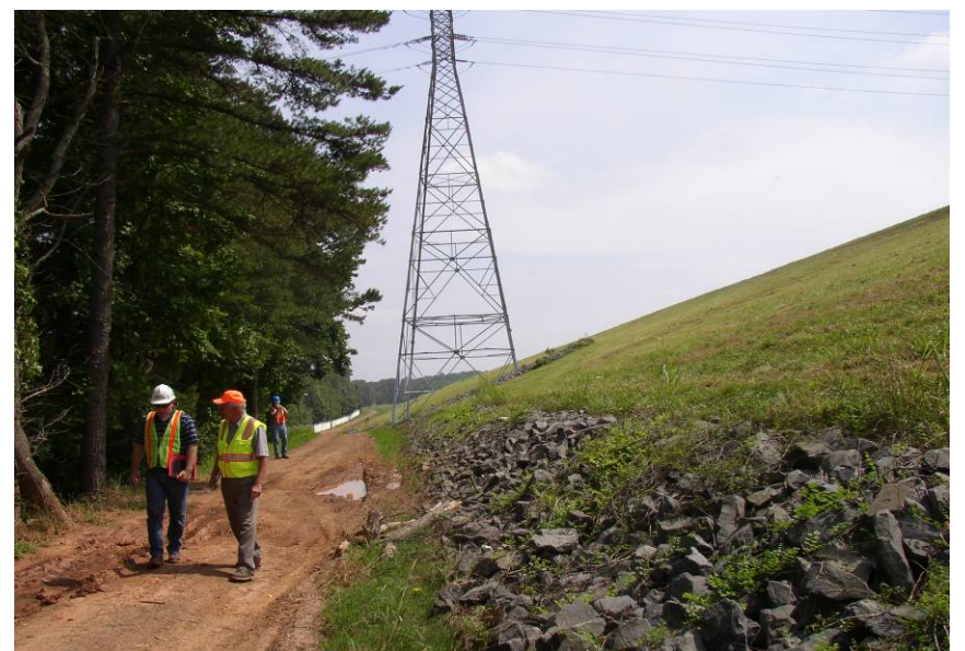
#40 Downstream Toe Road at North End of East Dike - Erosion
