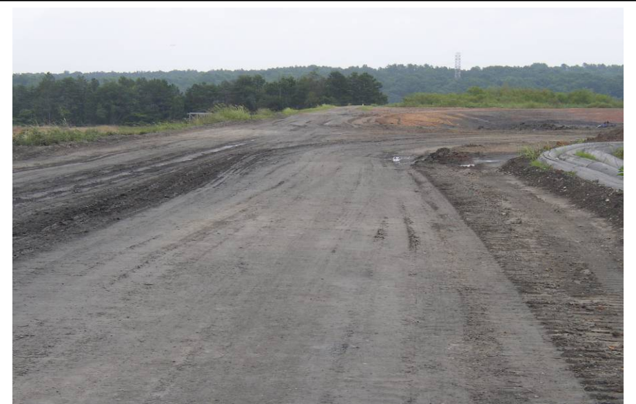
#51 Widened Crest in Cell 3 to Create Haul Road. Width Increased from 15 to about 45 Feet.
