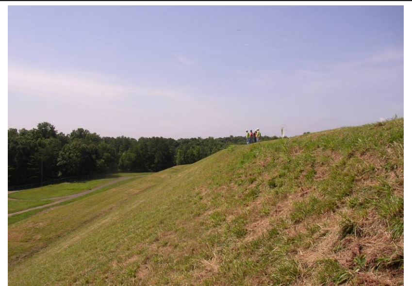
#10 Southern Downstream Slope of East Dike - Note Local Scarps in Upper Slope
