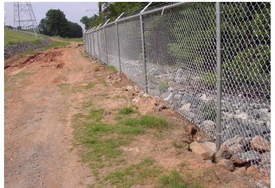
#39 Local Erosion / Rutting of Downstream Toe Road. Near Central Portion of East Dike
