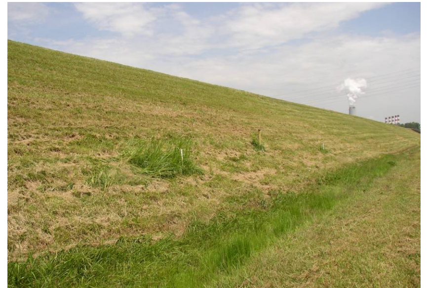
#26 Piezometers and Observation Wells Along Toe Stability Berm at South End of East Dike. (Note Standing Water at Toe)
