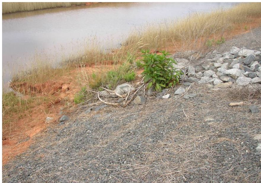
#46 Local Erosion @ Toe of Crushed Stone Drainage Material
