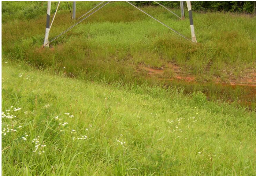
#68 Ponded Water Near Downstream Toe of North Dike
