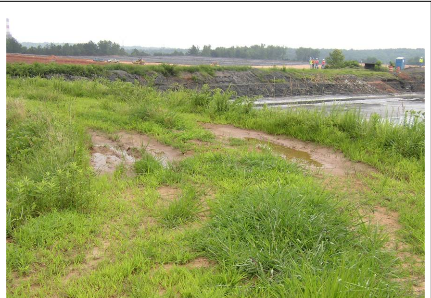
#71 Rutting in Crest at West End of North Dike
