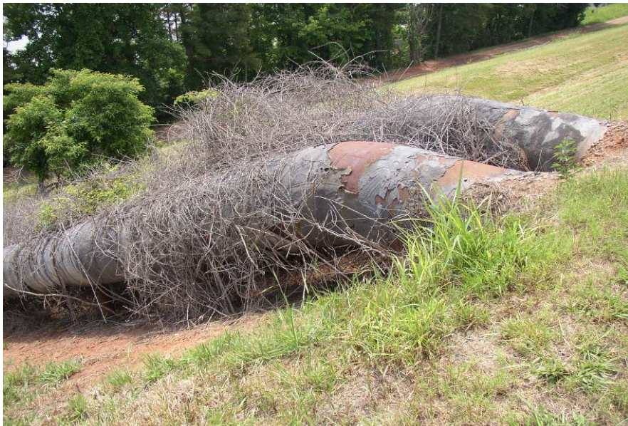
#16 Wastewater Sump Discharge Pipes @ Cell 3
