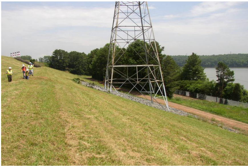
#23 Northern End of East Dike - Note Stability Berm Extends Over Transmission Tower
