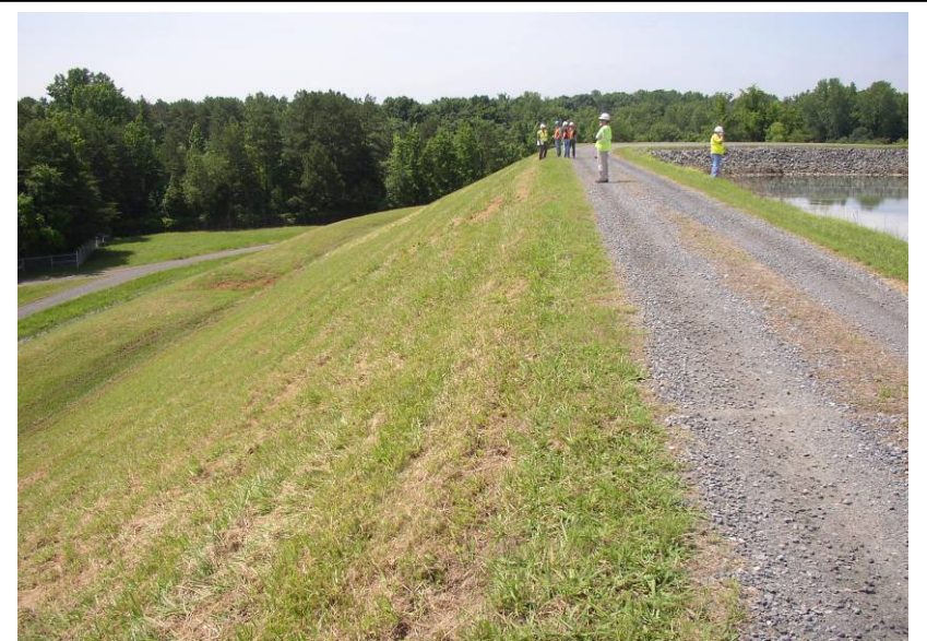
#9 Southern Portion of Crest & Downstream Slope of East Dike – Note Pooled Water on Berm
