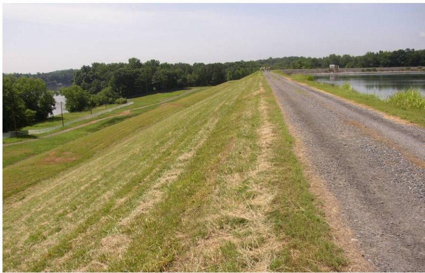
#11 Maximum Section Portion of East Dike – Note Wet Area at Toe and Local Berm Erosion
