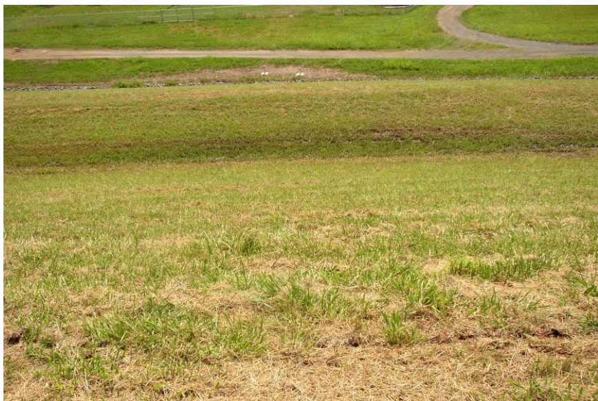
#8 Ponded Water on Bench of Downstream Stability Berm of East Dike
