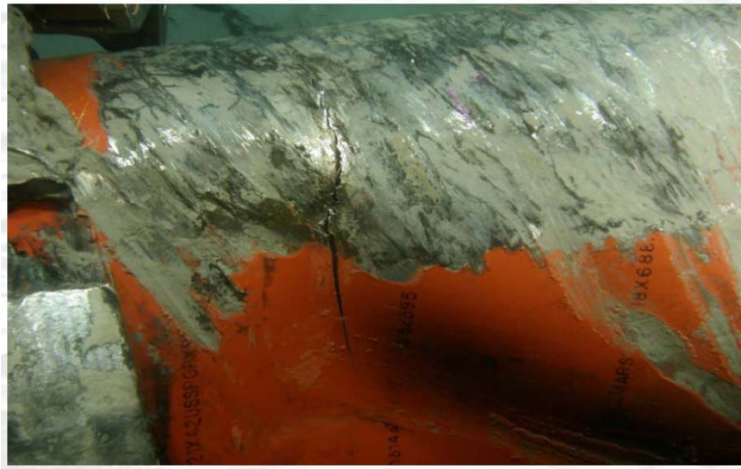
Figure 35 – MARS Pipeline Damage
