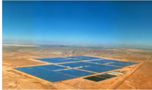
An aerial view of the parabolic trough arrays at Kramer Junction, California. The five facilities have a combined production capacity of 150 MW. (Credit: Gregory Kolb, Sandia National Laboratories)
