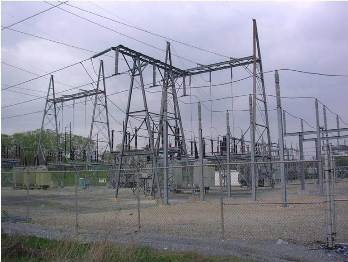
Figure 3.3: Pennsylvania Power & Light Electrical Substation in Columbia, PA
