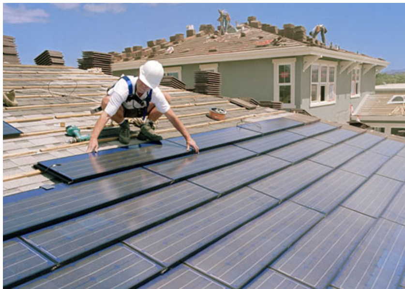
Figure 2.10: Roof integrated PVs and Solar Thermal Panels on a Maine Residence
