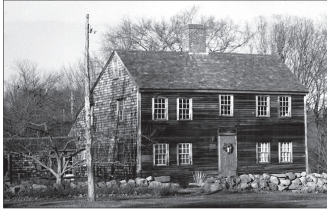
CPA funds have been used to shore up the foundation of Bedford's historic Job Lane House.
